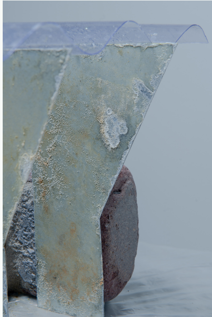
CORROSION OCCURS AS A RESULT OF CHEMICAL REACTIONS BETWEEN METAL AND ITS ENVIRONMENT, AFFECTING THE MATERIAL'S STRUCTURAL INTEGRITY.
